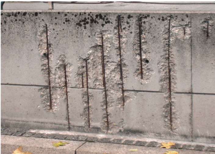
Corrosion of reinforced concrete following the use of deicing salts
